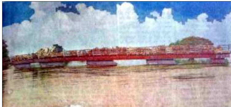
Fig 1: Broken-bridge in alamnagar on the Kosi River
